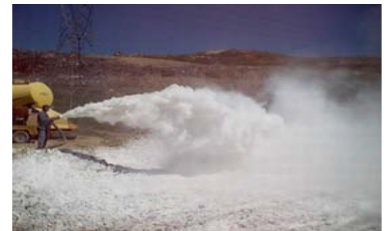
Covering over of a solid waste site with Alkeo-Hydrate disinfectant in powder
